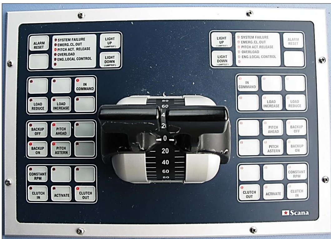
Figure 13. Closeup of bridge control panel order levers and command buttons.
