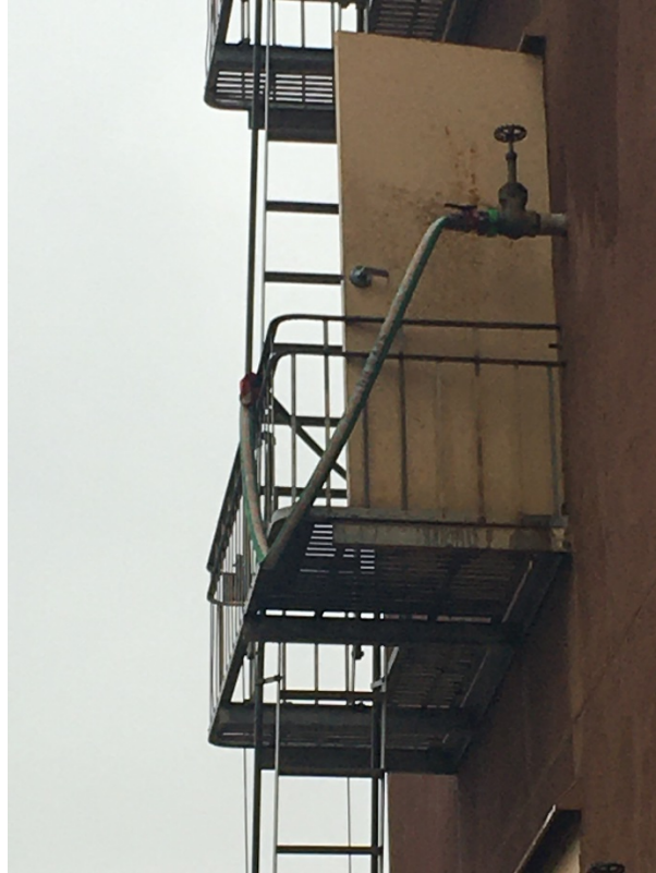
Close up view of the third floor fire escape and standpipe outlet
