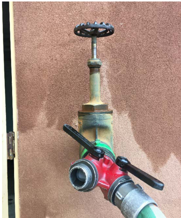
Standpipe outlet on third floor fire escape
