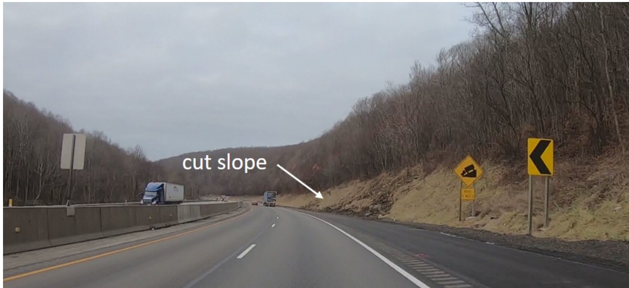
Figure 5. Frame from NTSB Daytime Drive-through Video Showing the Cut Slope
