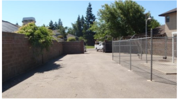
Alternate view of wine country lift station.
