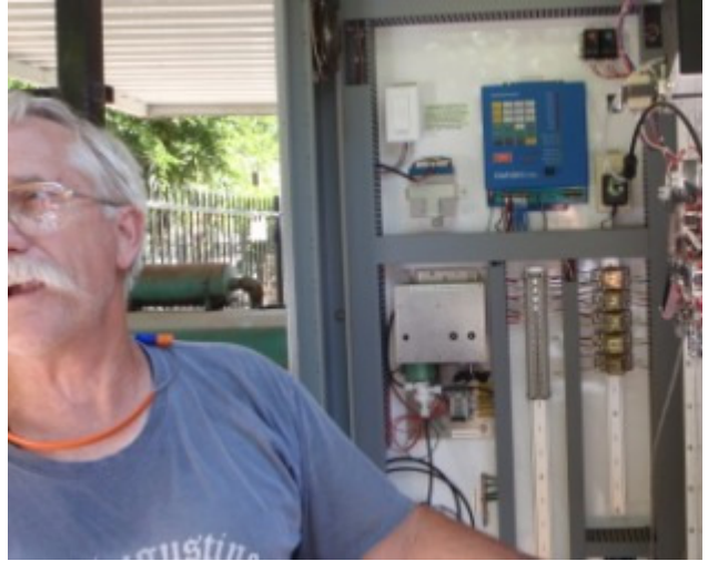
Lift station control panel being inspected by District collections staff at country club lift station.
