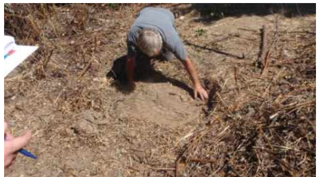
Manhole being inspected by District collections staff immediately adjacent to wine country lift station.
