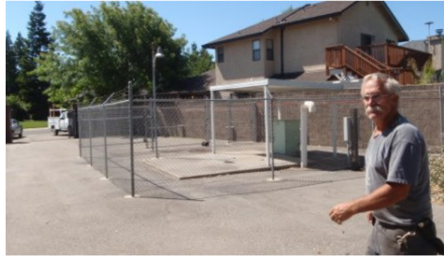
View of wine country lift station.
