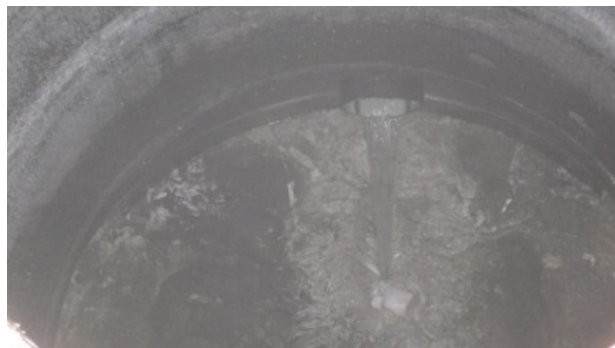
Alternate view of wet well at wine country lift station. Note accumulation of solids and grease inside wet well.
