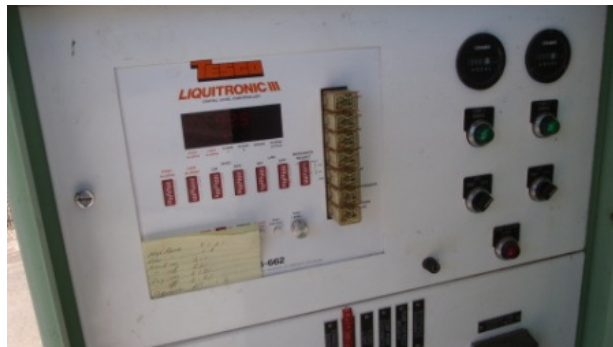
Alternate view of lift station control panel at wine country lift station. Note: alarm system inside panel not in use at this station.
