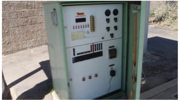
Lift station control panel at wine country lift station. Note: alarm system inside panel not in use at this station.
