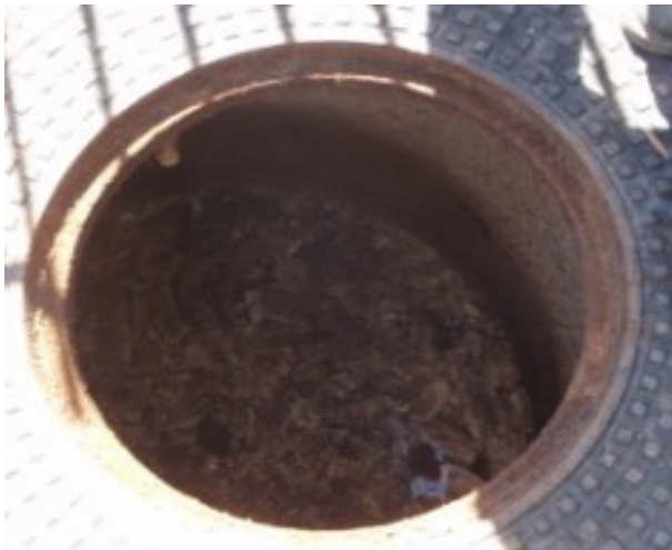
Close up view of wet well at country club lift station. Note accumulation of solids/grease.
