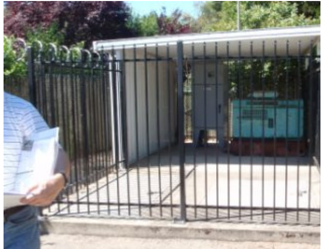
Outside view and perimeter fencing at country club lift station.
