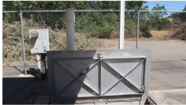
Dry well door opened at wine country lift station.
