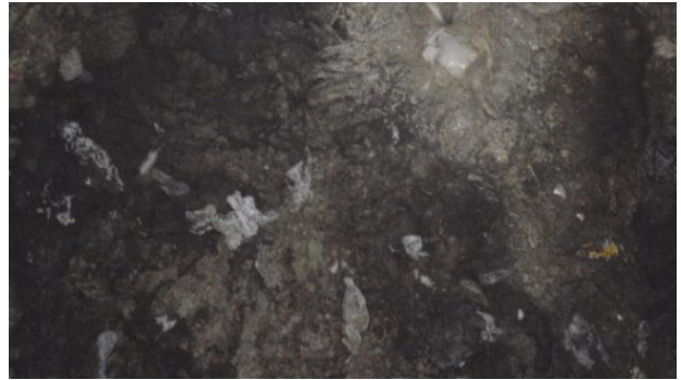
Alternate view of view of wet well at wine country lift station. Note accumulation of solids and grease inside wet well.
