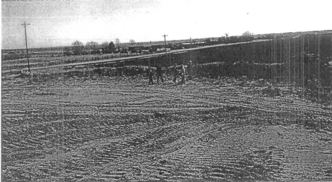
Photo 3: View to the east-northeast of paint dumping location, roughly where the group of people are standing.
